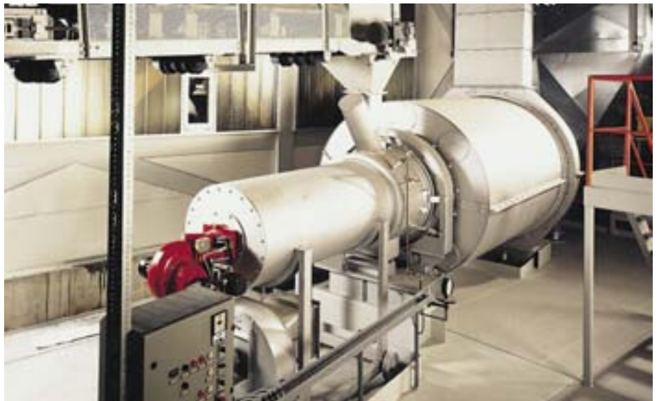
Triplex dryer with hot gas generator
